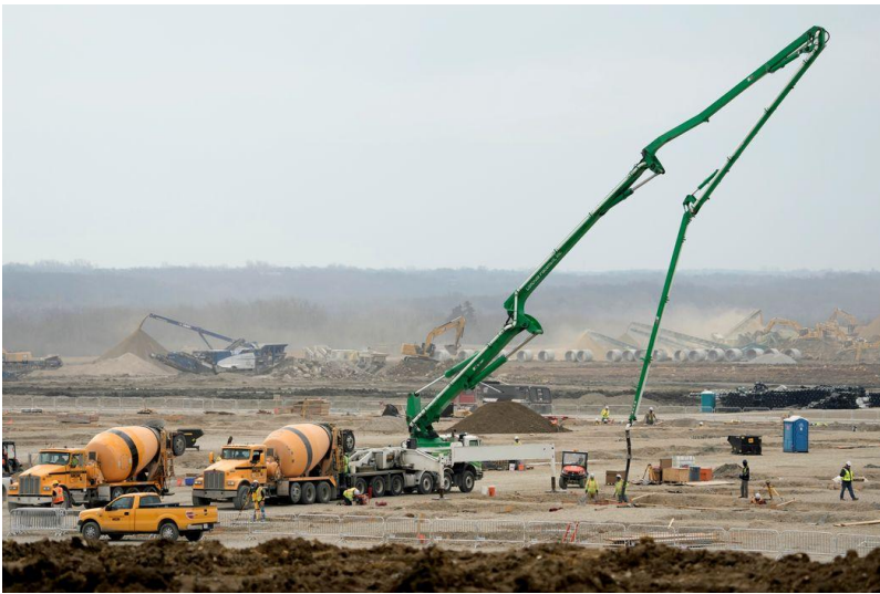
Workers prepare the site of a Panasonic EV battery plant near DeSoto, Kan. PHOTO: CHARLIE RIEDEL/ASSOCIATED PRESS
